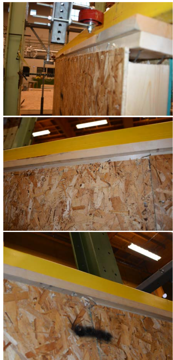
Figure 10. Failure modes for multiple-panel SIP wall without openings.
